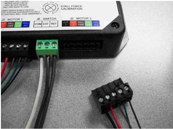
Motor connection at board
